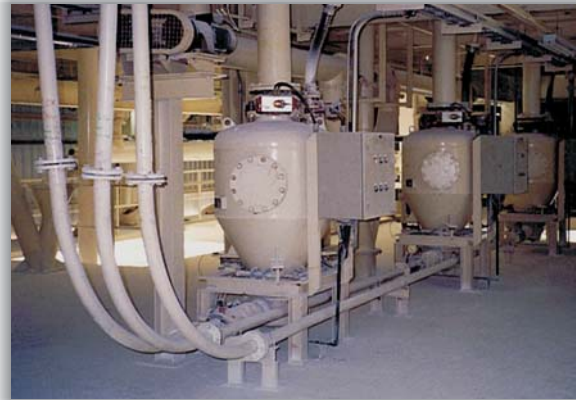
pressure vessel conveying
