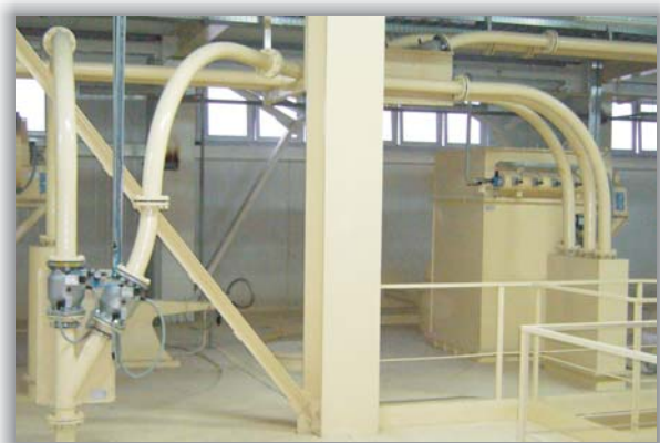
pipe diverter, dust separator
